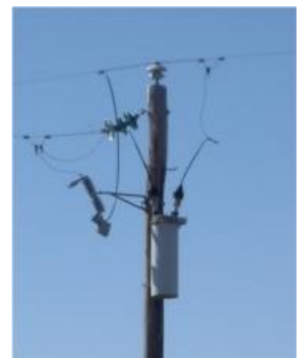
A 240V tap on a Single Wire Power line
